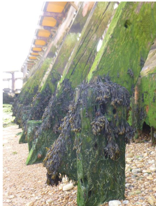
Base of wooden jetty showing epiphytic community within tidal zone © Ben Kimpton.
