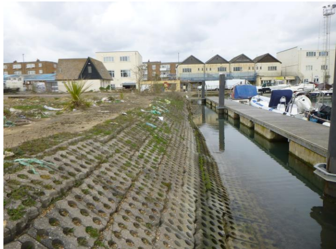
Concrete blockwork revetment around eastern edge of vacant land at Lady Bee Marina. Forms part of SS3 © TEC.
